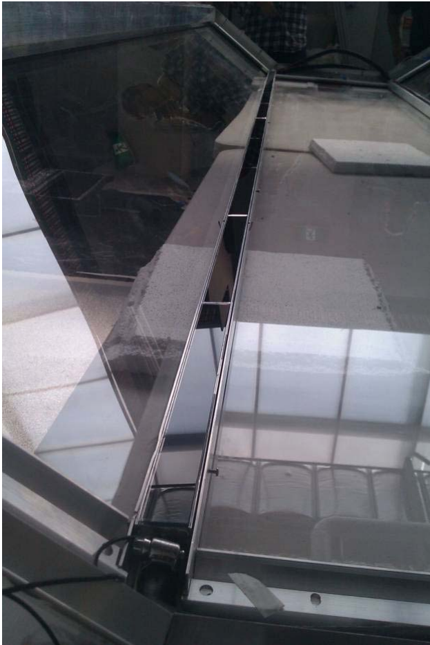
Fig. 6: A completed receiver mounted in open box, with plumbing and electrical interconnection completed.
