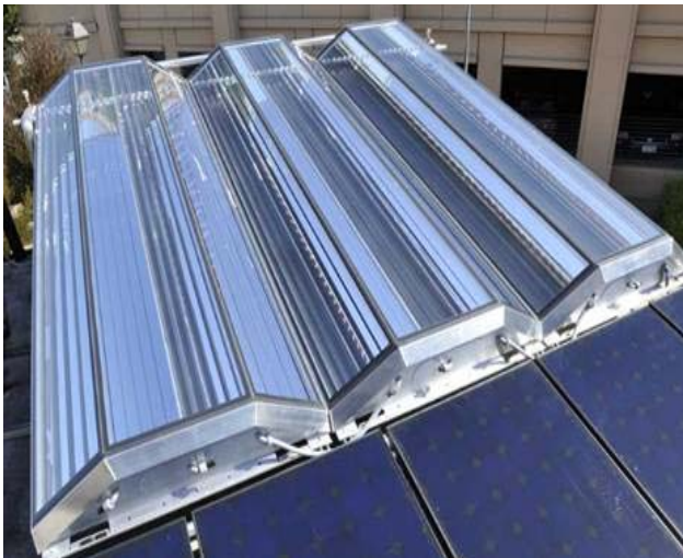
Fig 1: Three MCT units mounted on a demonstration rooftop. The light-weight, low area-loading MCT systems were mounted on the same supporting frame as the surrounding flat-plate PV panels.
